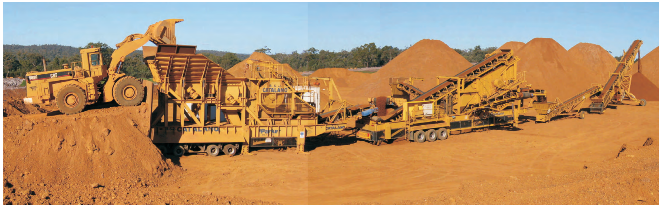
Mobile crushing plant used by Catalano to crush gravel. The proposed plant will be of a similar scale
